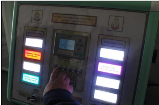
Fig. 10-c. O.C. Protection Unit in operation
