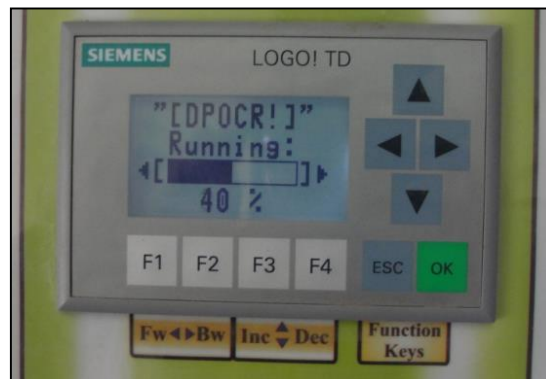
Fig. 10-b. HMI of the PLC O.C. protection unit
